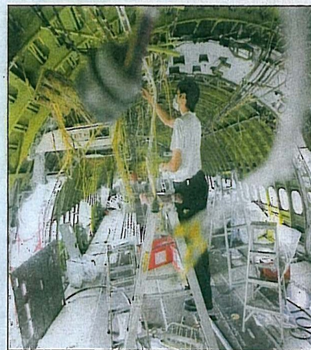
An aerospace technician rewiring the interior of a passenger plane to convert it into a freighter aircraft. The aviation and aerospace sector employs more than 18,000 people and has been growing steadily, driven by Asian demand. ST FILE PHOTO
